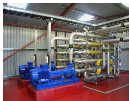
b) Plant for membrane water filtration.
