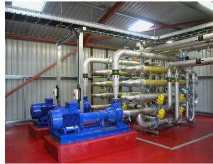
b) Plant for membrane water filtration.
